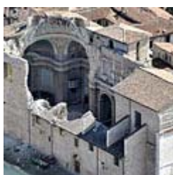
A damaged church in L'Aquila
